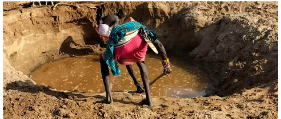
A ramp being dug by our team, everybody can safely access the
