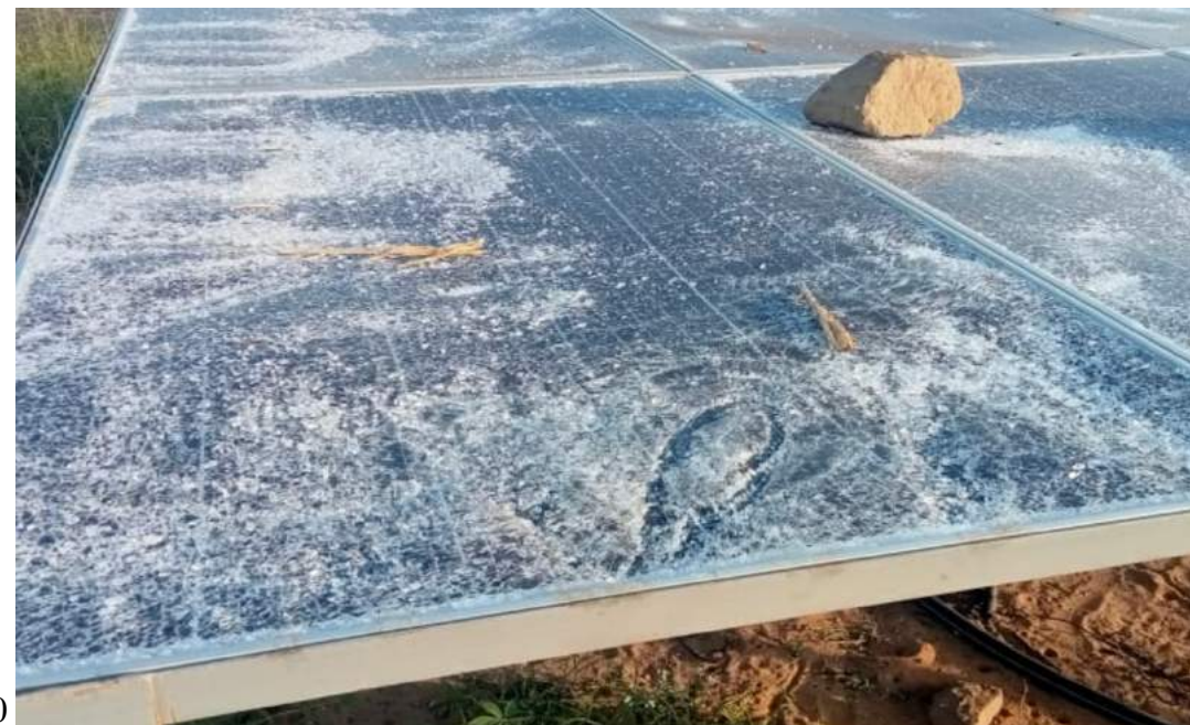
Murran water project damage
